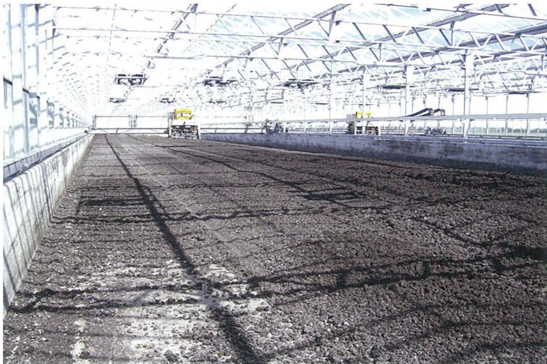
Figure 6: Photo of inside the Selwyn District Secondary Solids Drying Facility
