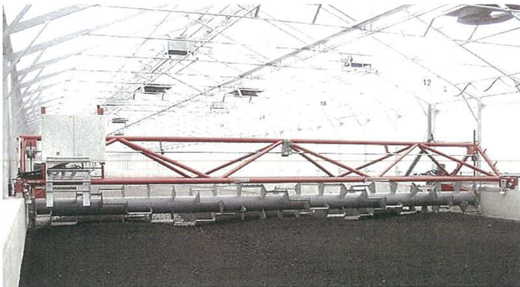
Figure 4: Picture of an operating Solar Drying Facility similar to that proposed by the applicant
